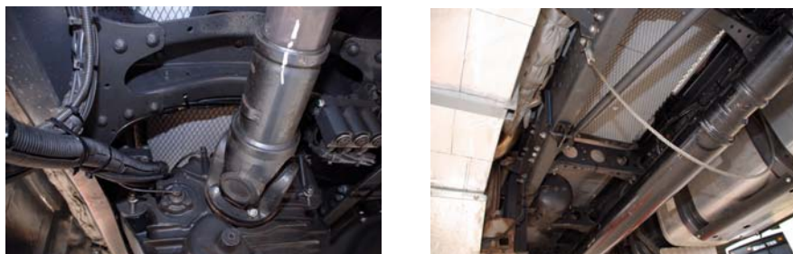
Fig 13. The installation of Megasorber FG50 with expanded metal mesh above the transfer case.
